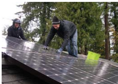
Solar energy can become an increasingly important part of Oregon’s effort to reduce global warming pollution, while simultaneously becoming a substantial force in our economy. Credit: Solar Oregon
