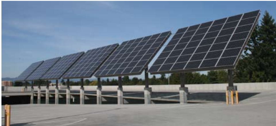
Solar photovoltaic panels—like these installed on top of a parking garage in Hillsboro—turn sunlight into electricity. Credit: Flickr user born1945
